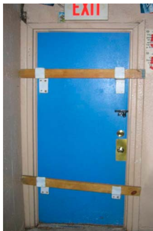
Locked and blocked exit
