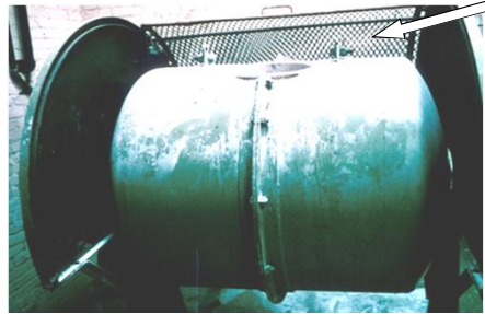
Interlocked guard on revolving drum
