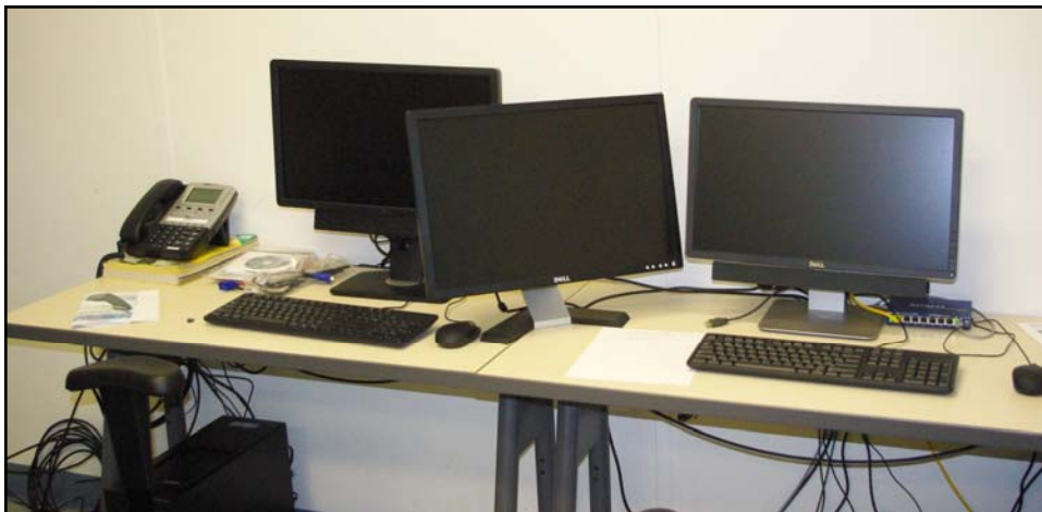
Computers tied to alarm systems and building control system; land-line telephone
